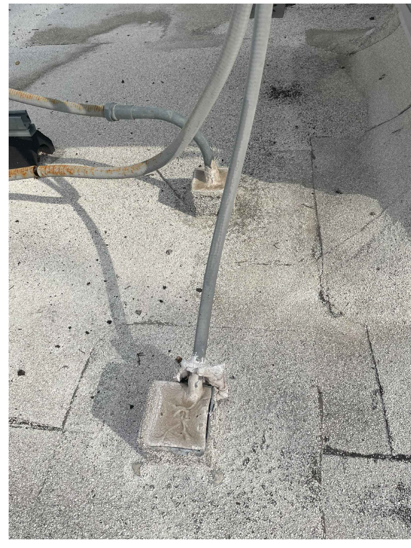
Electrical Roof Penetration • Remove sealant and mastic at conduit and unistrut roof penetration. • Verify integrity of modified bitumen roofing membrane at penetration curb. • Reseal penetrations and apply roof sealant. • Install new weatherseal, cover and gasket at electrical outlet and j-box. Refer to 02/A2.05, 03/A2.05.
