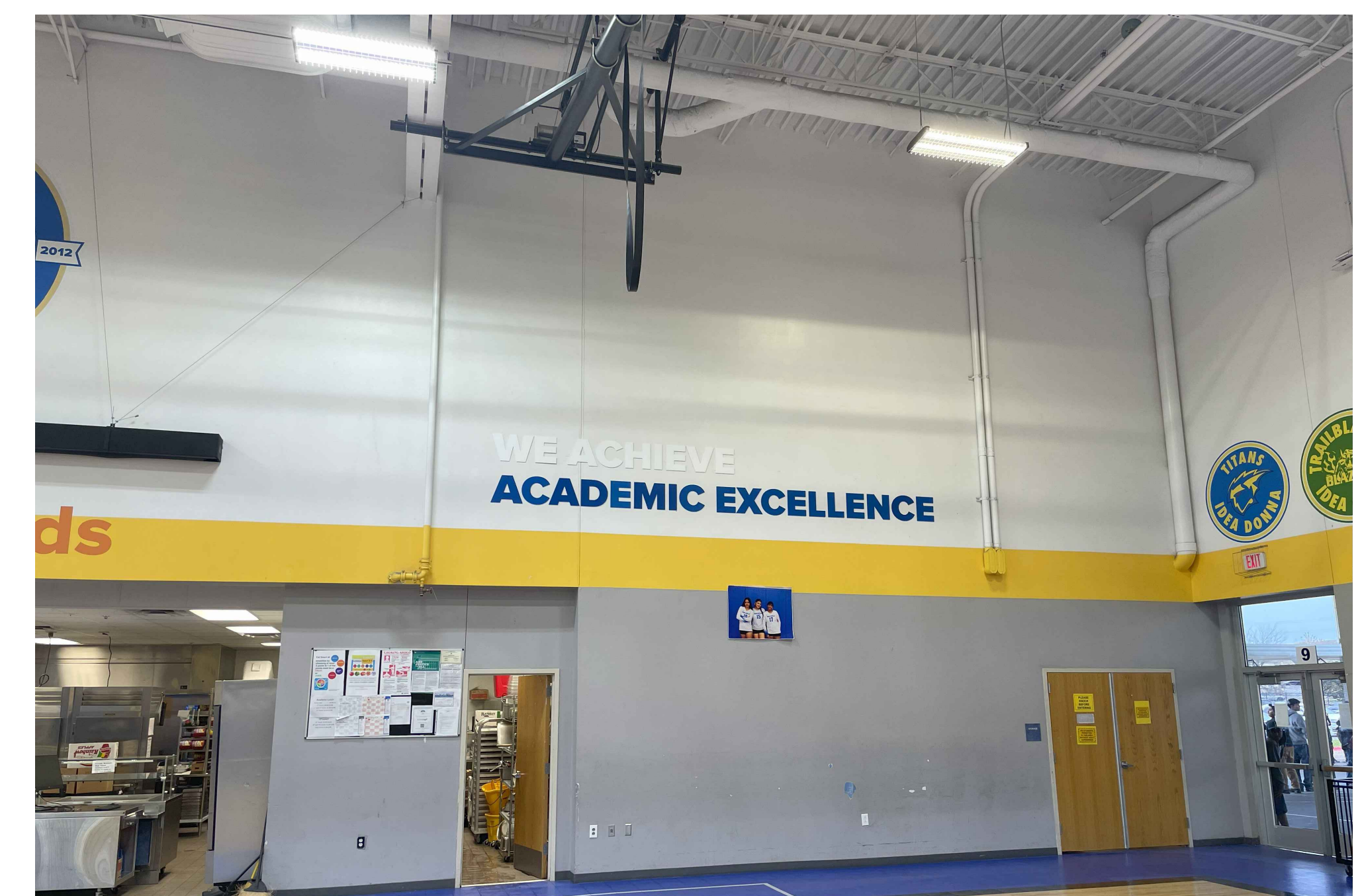
PICTURE #1 - ROUTING OF ROOF DRAIN LINE
