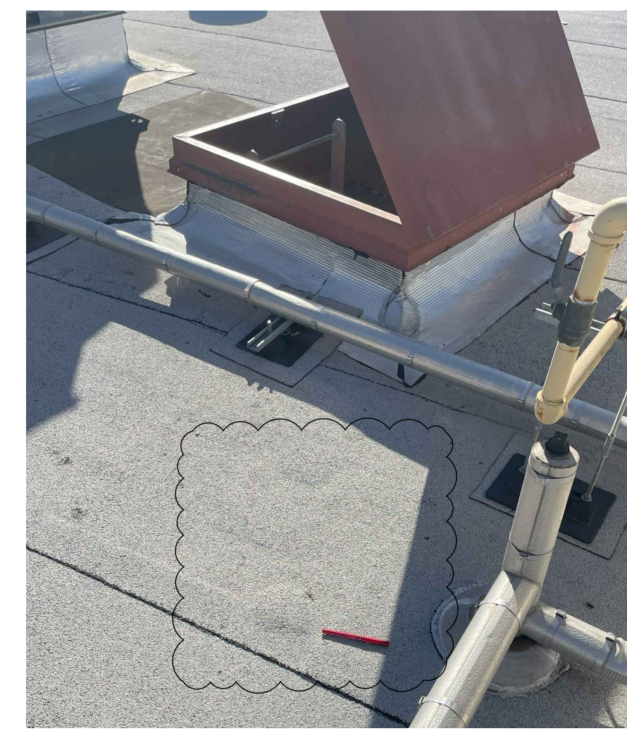
Roof Membrane Bubbles • Remove flashing transition membrane at parapet wall. • Verify integrity of modified bitumen roofing membrane and underlayment. • Install new membrane repair and accessories.
