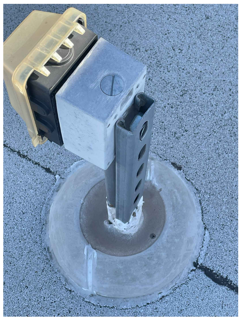
Electrical Roof Penetration • Remove sealant and mastic at conduit and unistrut roof penetration. • Verify integrity of modified bitumen roofing membrane at penetration curb. • Reseal penetrations and apply roof sealant. • Install new weatherseal, cover and gasket at electrical outlet and j-box.
