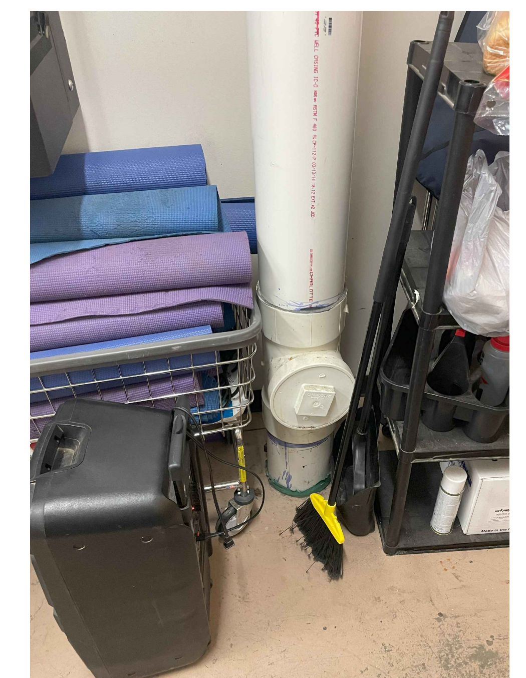
PICTURE #3 - ROOF DRAIN LINE FLOOR PENETRATION
