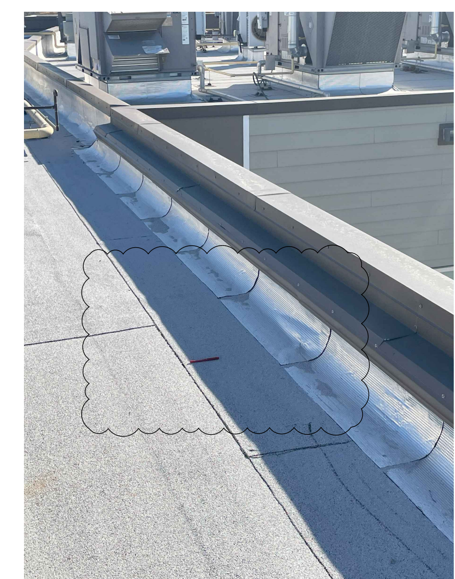
Roofing and Flashing Transition at Parapet Wall • Remove flashing transition membrane at parapet wall. • Verify integrity of modified bitumen roofing membrane and cant strip. • Install new membrane and counterflashing accessories.
